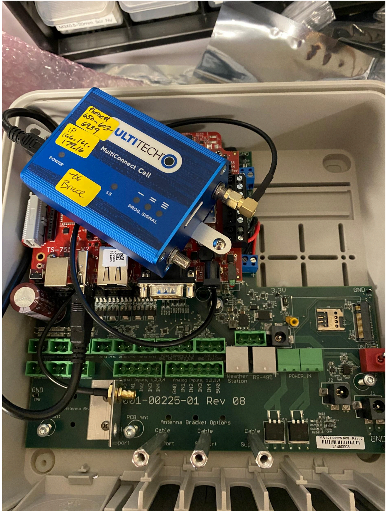
Figure 1.1: Water pump sensor module Assembly
